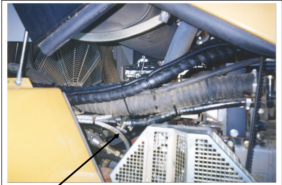
Heater shut-off tap installed in 5/8" heater line
